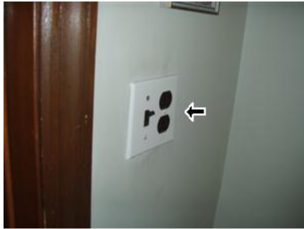
5.5 Picture 2 rec. GFCI
