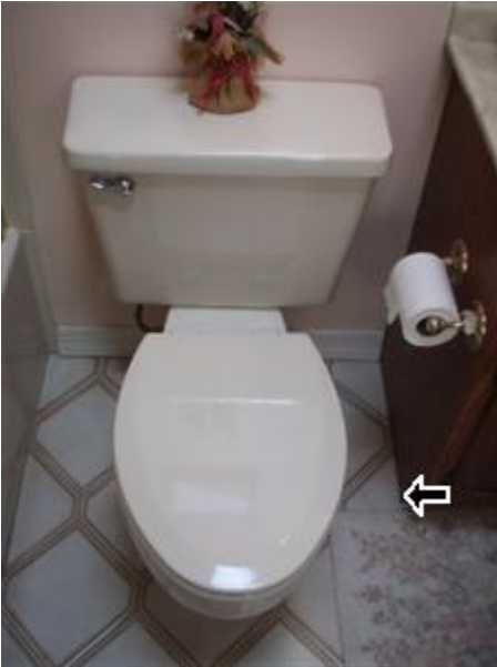
4.0 Picture 3 loose toilet.
