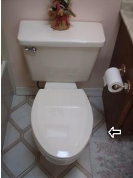
4.0 Picture 3 loose toilet.
